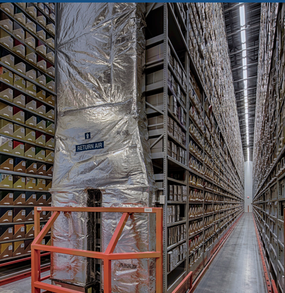
More efficient climate-control equipment in the three units has saved the WRLC $100,000 in energy costs in less than a year.
