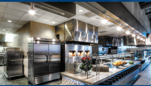
The cafeteria in the West Village Commons includes high-efficiency lighting and commercial kitchen equipment.
