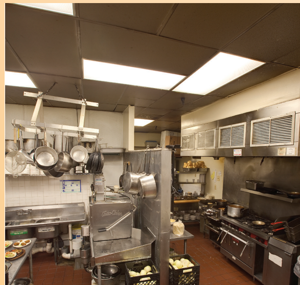
New lighting in the kitchen provides a brighter and, therefore, safer working environment for restaurant staff.
