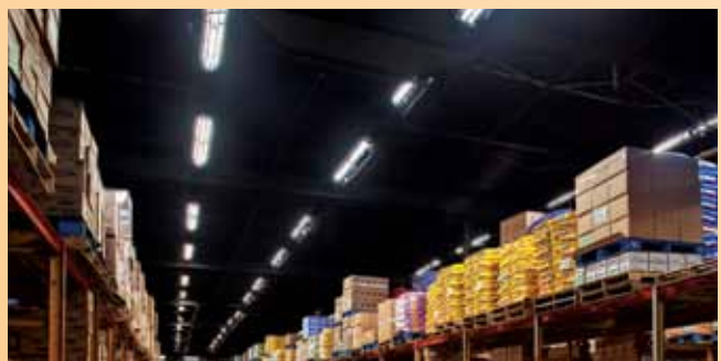
Upgrading to energy-efficient fixtures in the distribution center reduced energy use while improving lighting quality.
