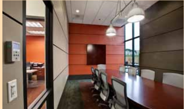
Mars installed high-performance lighting and occupancy sensors in its new corporate offices in Rosedale.
