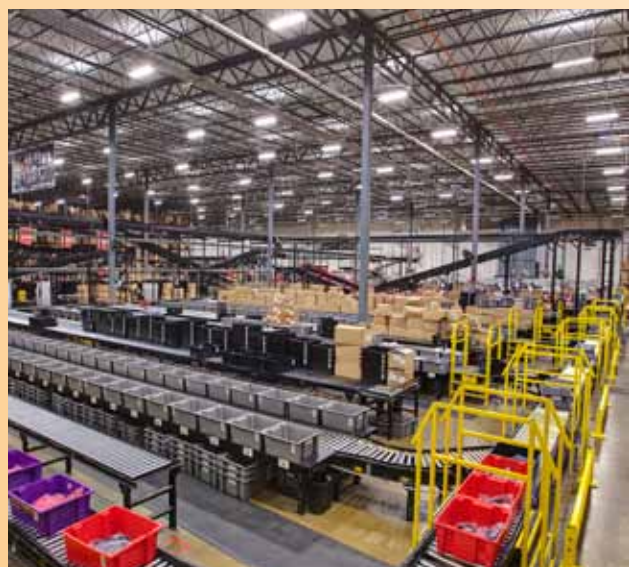
Under Armour’s 1010 Swan Creek Drive facility installed new lighting and occupancy sensors
